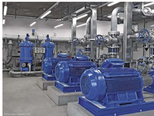
Pump station Dappler 741
